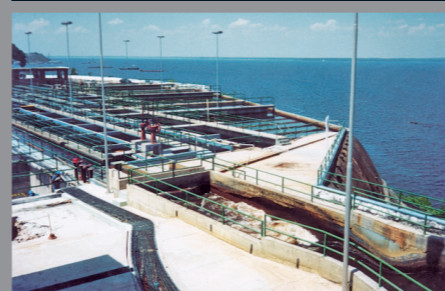
Ponta Do Ismael Water Treatment Plant, Brazil
