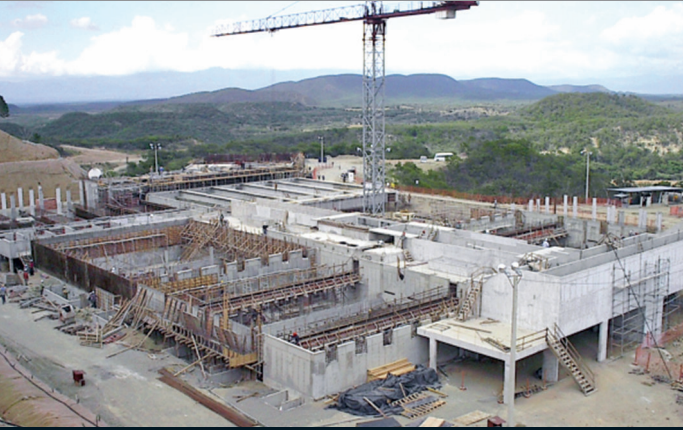
Mao Point Wastewater Treatment Plant, Dominican Republic
