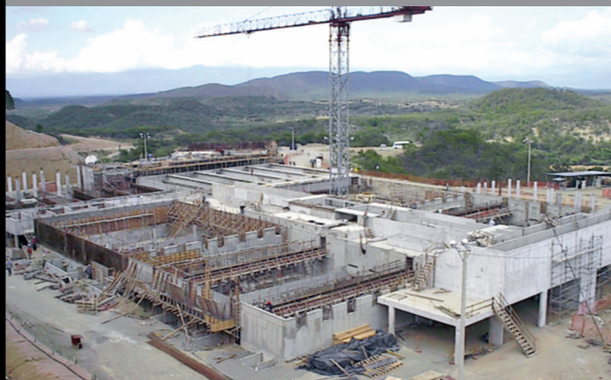
Mao Point Wastewater Treatment Plant, Dominican Republic
