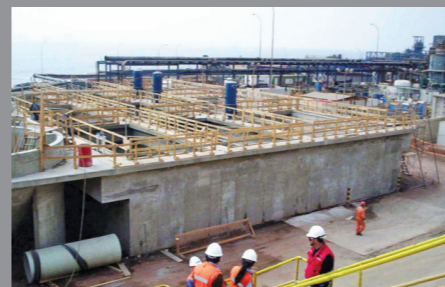
Reverse Osmosis Desalination Plant, Chile
