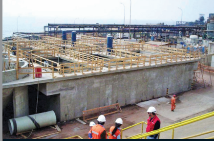
Reverse Osmosis Desalination Plant, Chile
