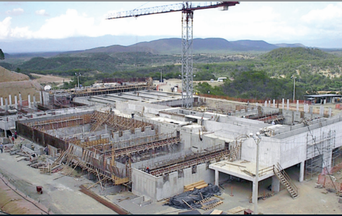
Mao Point Wastewater Treatment Plant, Dominican Republic
