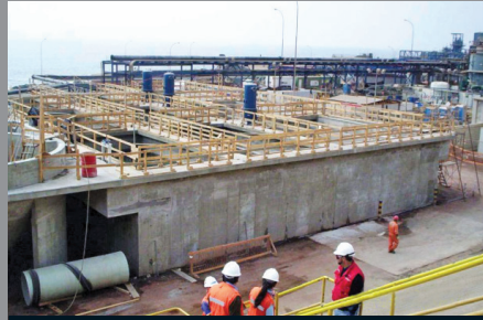
Reverse Osmosis Desalination Plant, Chile
